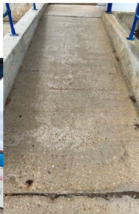
Uneven surface and exterior of unit
