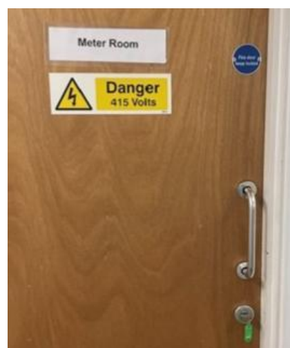
Concern: key left in door of meter room
