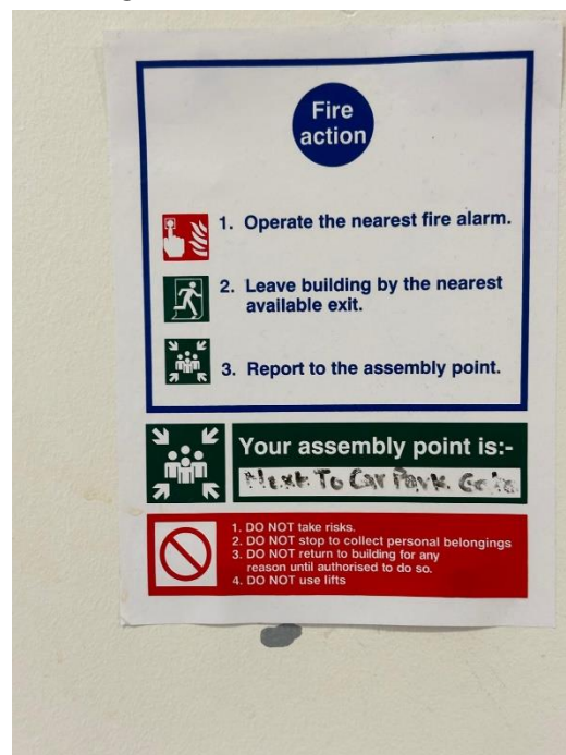
Figure 3: The fire safety information was worn and required maintenance.
