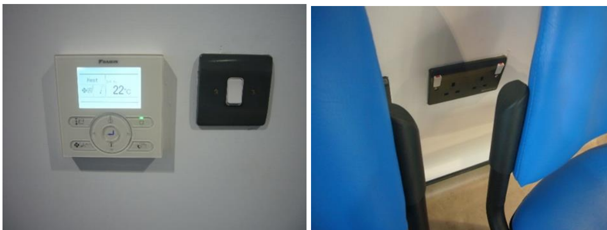
Air conditioning controls and plug sockets
