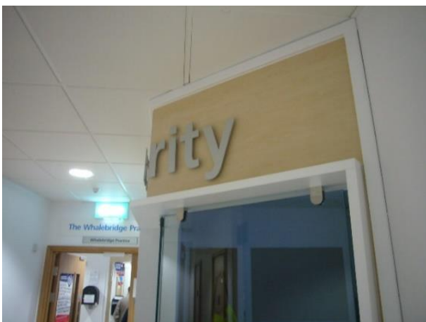
The security desk sign cannot be read in full from the main entrance
